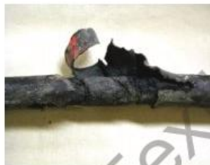
Fig: 15.23 Over heating of a cable
